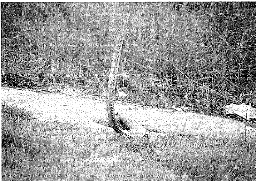
INTOLERABLE - OBJECT MARKER SEVERELY DAMAGED, NOT VISIBLE, OR MISSING
