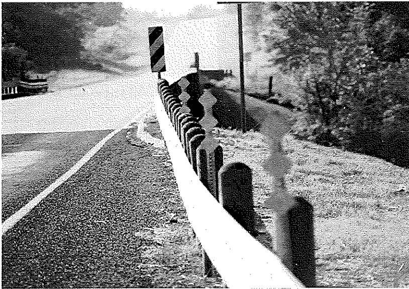
DESIRABLE - OBJECT MARKER CORRECT AND CLEARLY VISIBLE
